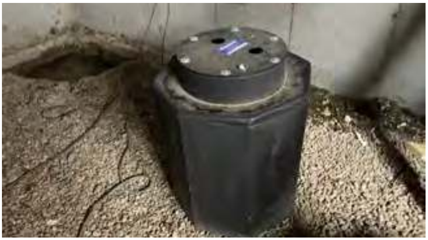
Photo: A sump pump system prior to installation in the sump pit.
