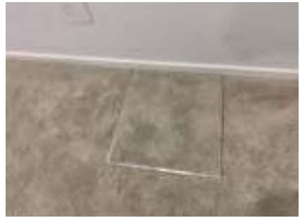
Photo: A backwater valve location with the floor cover over it.
