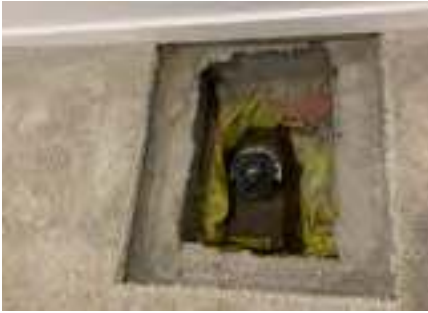
Photo: A backwater valve located in the basement of a home.
