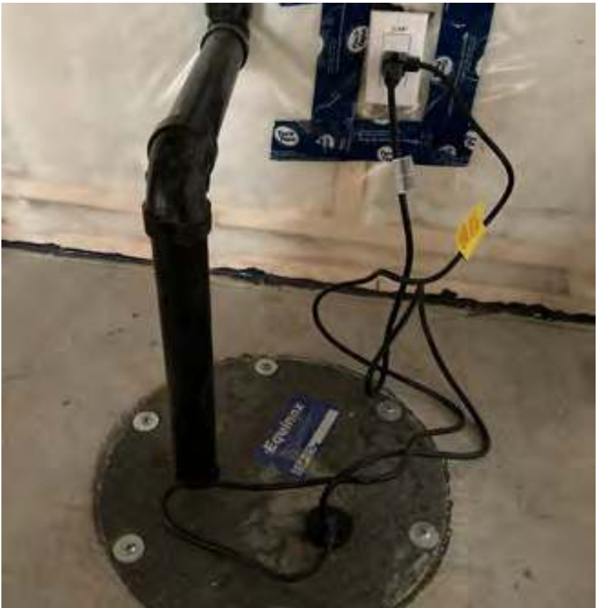
Photo: A properly installed sump pump system.
