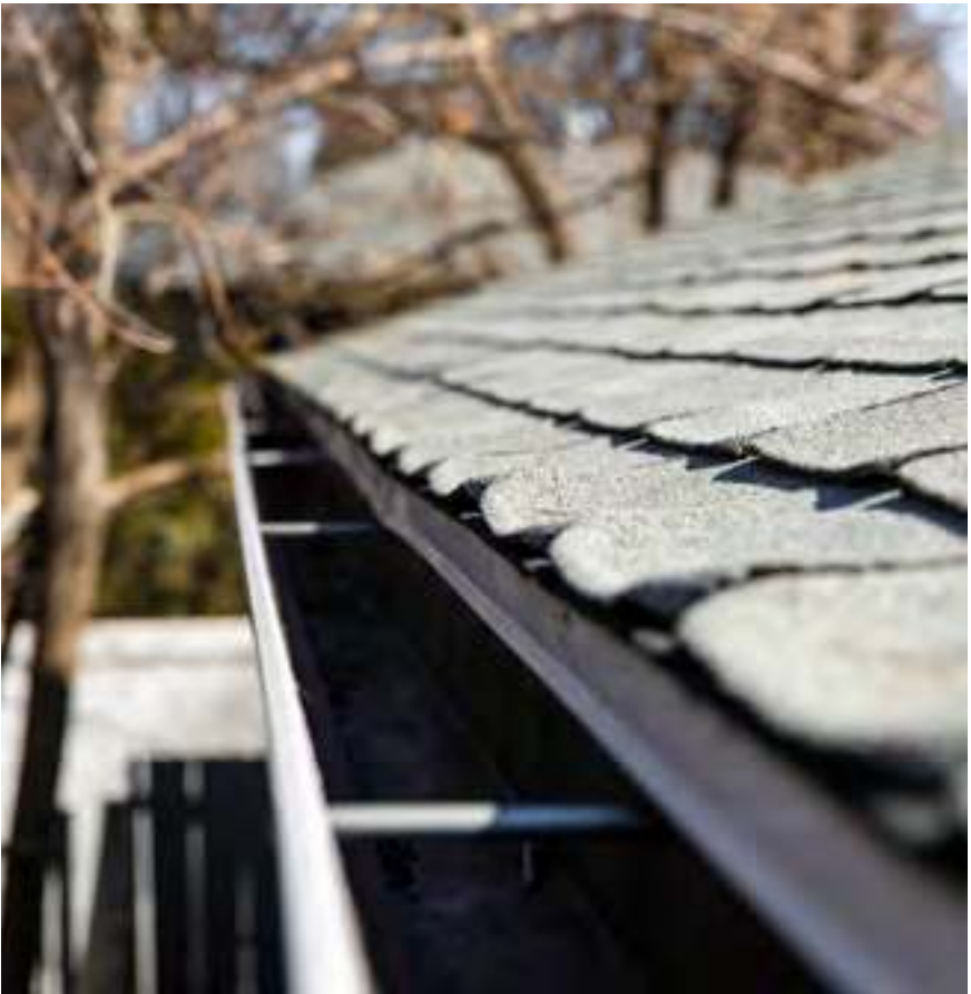
Photo: Your first line of defense against the rain and snow is the roof and eavestrough system. Make sure these are in good repair.
