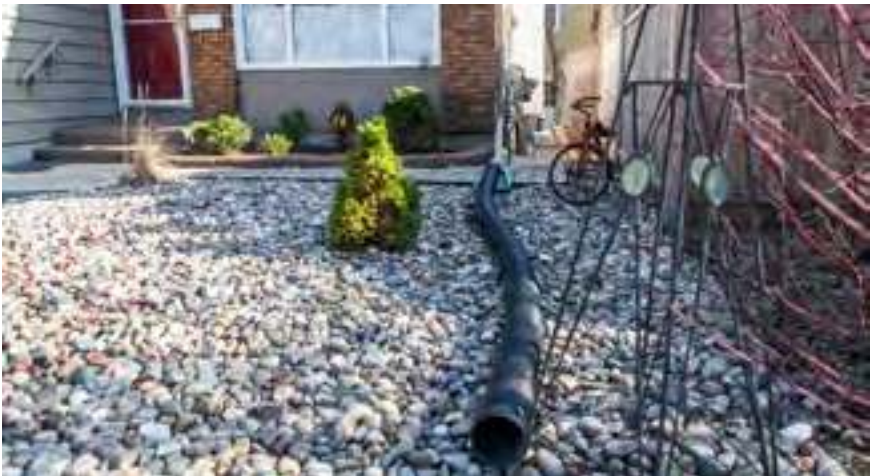
Photo: Downspout extensions should direct the water away from your home, but not into your neighbour's property.
