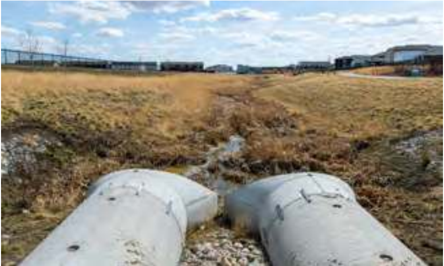
Photo: Storm culverts allow for water to cross roadways and other obstacles.
