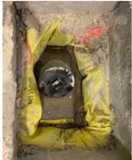
Photo: A backwater valve in a home.
